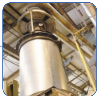
Heat energy recovery unit at the Escol factory
